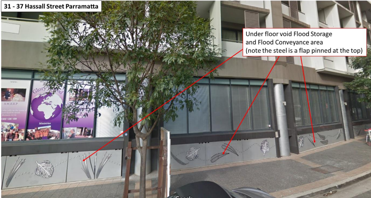
Plate 8 Example of under floor void flood storage and conveyance (31 - 37 Hassall St Parramatta)
